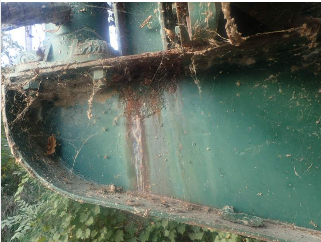
Long bracket, corrosion of rail post connection and top plate of bracket. Blistering of bracket web.
