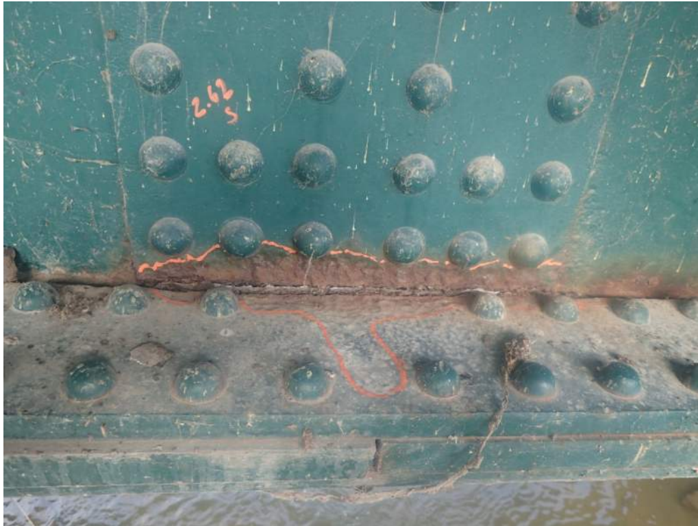
Closeup of exterior beam splice plate corrosion and section loss
